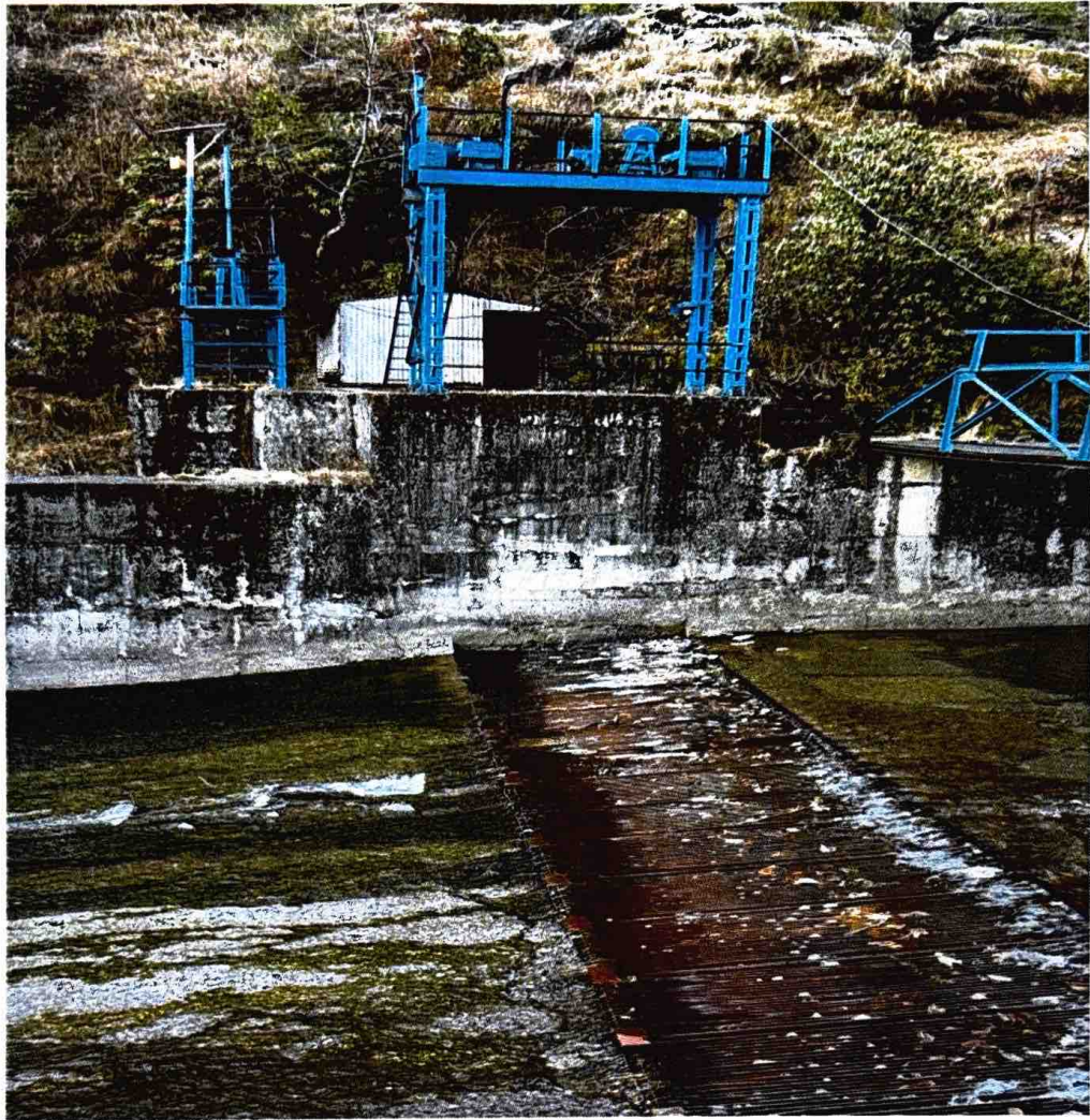
Release of flow from project to river
